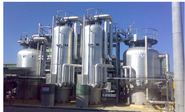
Fig 5 Picture of CambiTHP™ in WWTP Brisbane
