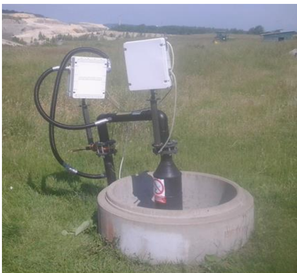
Figure 3: Continuous monitoring unit installed at landfill gas extraction well
