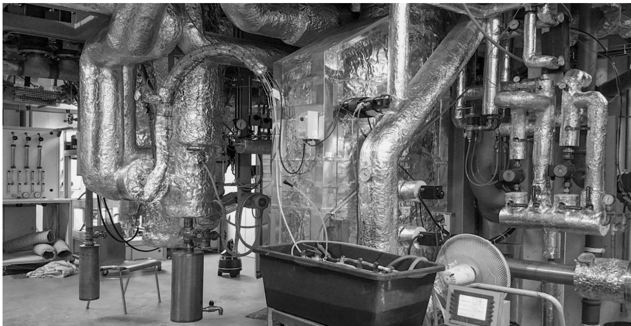
Figure 2. Actual pilot scale of online product gas measurement with insulation-assembled components
