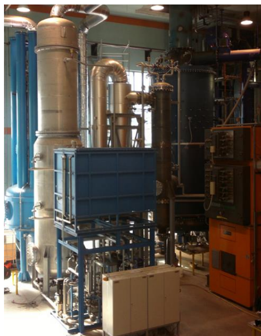
Obr. 18 Jednotka technologie Pyrox Fig. 18 Gasification equipment - Pyrox
